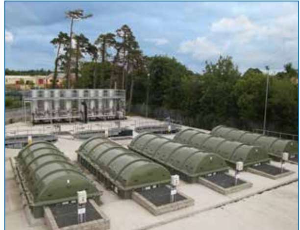
2000 PE Wastewater Treatment Plant.
